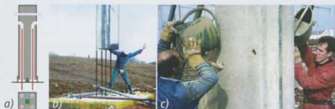
Fig. 2 Mounting of the prefabricated column on the concrete foundation – a system widely applied in Belgium, a) concrete reinforcement on which carrying supports are placed protrude from the concrete foundation, b) necks are placed on the reinforcement protruding from the concrete foundation or the preceding prefab element, c) necks with reinforcement and incurred hollows are filled with thin, non-shrinking filler
